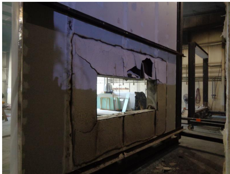
Photo No. 13 First Floor Interior Gypsum (Post-Test)
