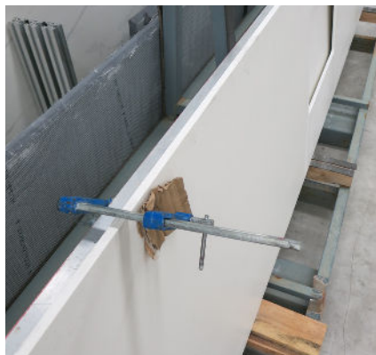
Image 3: Plank in the backside of the slab
